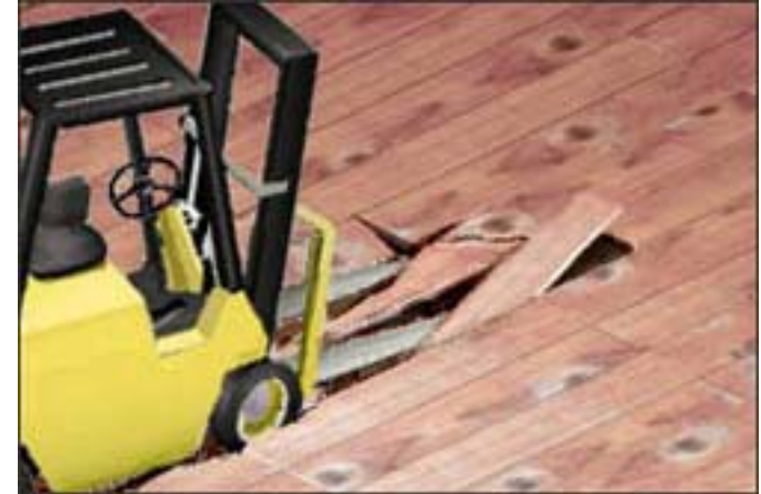
Forklift weight exceeded the load limit of the flooring.
